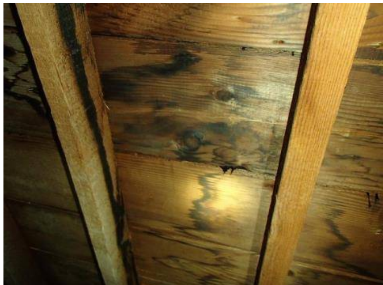
Needs Attention: There are areas of stains on the framing lumber these appear old and may be from a previous roof leak.
