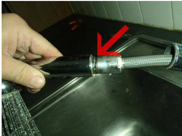
Not Acceptable: The kitchen faucet leaks at the base of the line / handle connection.
